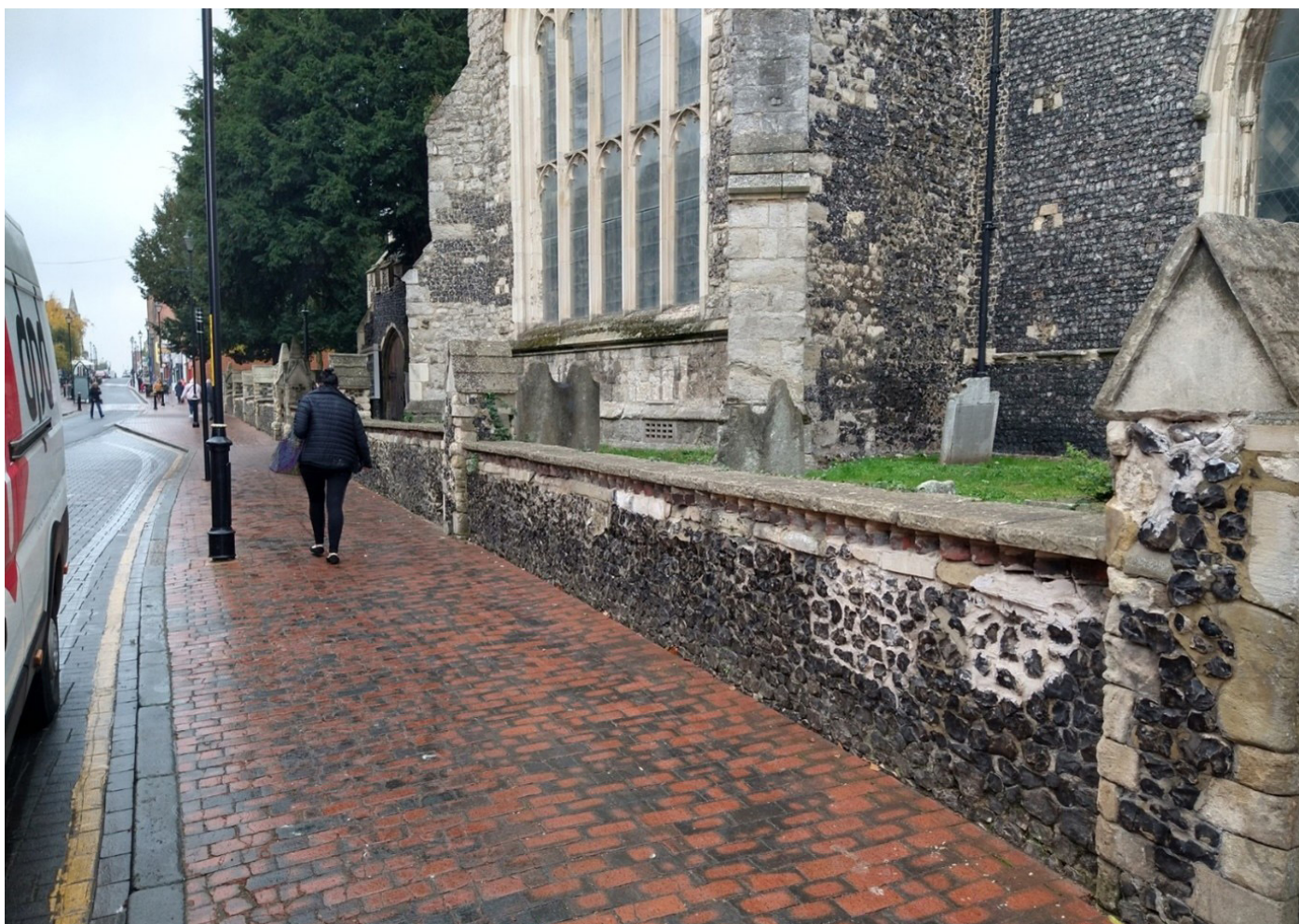
High Street public realm and boundary to St Michael's Church in need of repair
